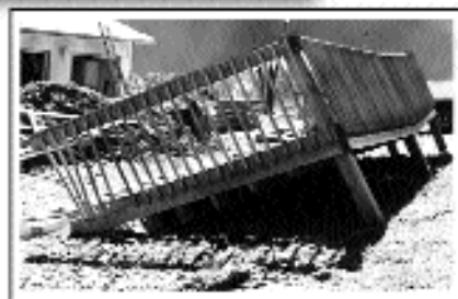
Photos of brand-new, fine house destroyed due to a bad foundation.
